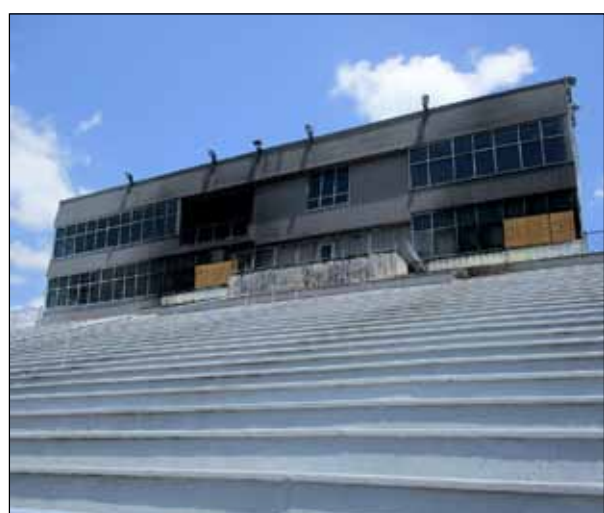
Investigation into the fire at the football stadium determined the blaze was started by the sun reflecting off the glass of the press box which ignited the special covers on the vinyl VIP seats in front of the press box.
