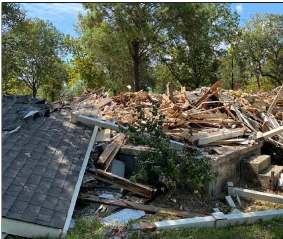
The rubble is from condemned buildings at the Sabine Park Apartments between First and Second Streets in the Old Orange Historic District. Last week the demolition began on the wood-frame one, and two-story buildings. The city is paying the Lark Group $145,000 to demolish nine of the complex's buildings. A lien for the amount will be added to the property so the city can be paid back.
